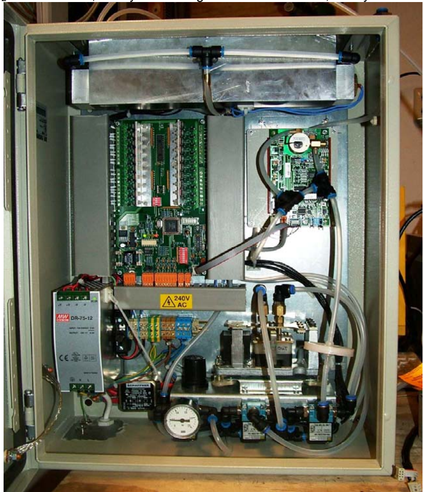
Fig. 1: The CO 2 substation.
